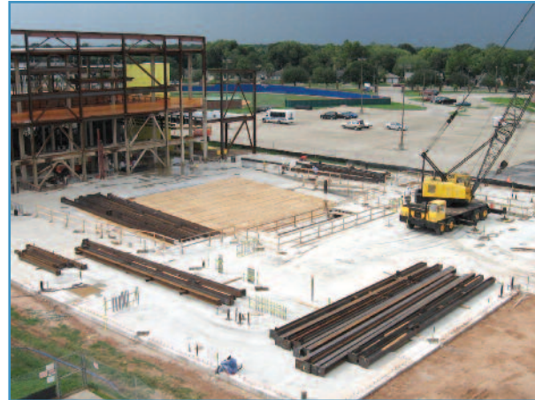
Under construction: At this point, most of the budget is committed and it's too late for significant changes.
